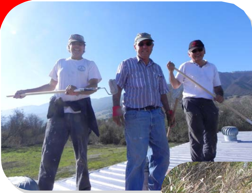
Left—introducing the roofing crew; Joe Francis, Chuck Bosso and Richard Tanaka. Swab the deck, boys!
